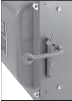
Cover Interlock Key Opening on 82,000 Line
