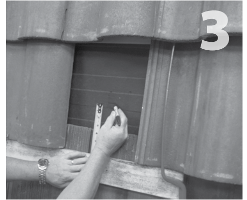
Use a straight edge and measure up 6 5/8" from bottom of tiles to center of the mount over the center of rafter.
