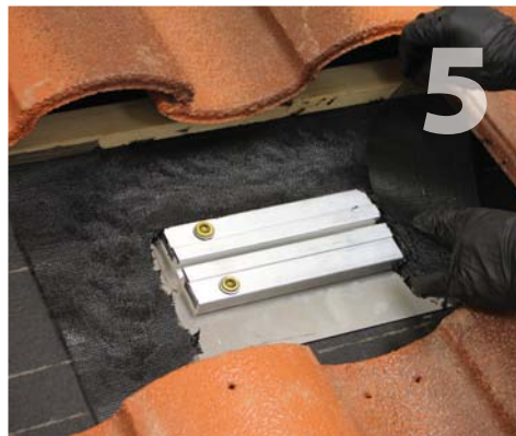
While cement is still wet apply 3 pieces of roof repair fabric strips where felt paper and flashing meet – a 16" strip along the top, and a 9½" strip along each side.
