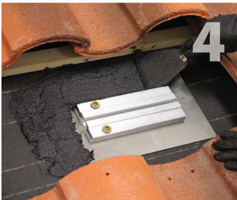
Apply \frac{1}{8} " thick layer of roofing cement around the top and sides of the sub-flashing with at least 2" extending past the sides of the flashing onto the felt.
