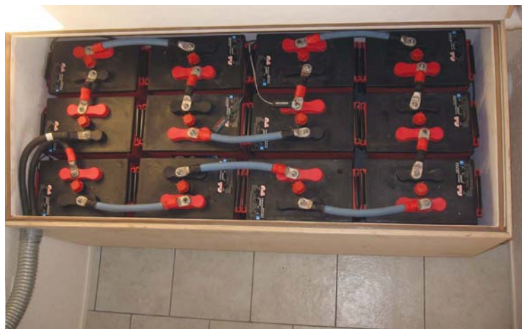
A single 24 V string of 2 V flooded cells has about the same size and capacity as the three strings of L-16s, but with fewer cells to water and fewer interconnects.
