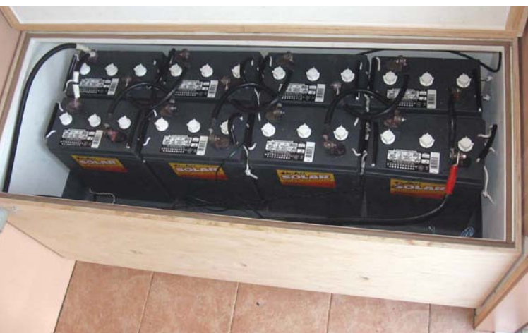
Two paralleled 24 V strings of 6 V Deka L-16 batteries in an enclosure sized for three strings, interconnected and arranged to allow easy access to the electrolyte caps for maintenance.
